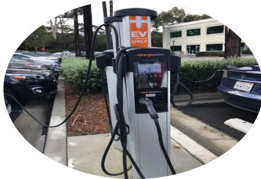
Electric Vehicle Charging Stations
