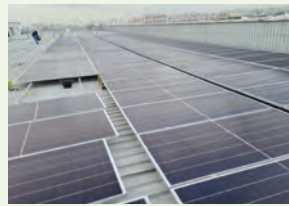
Solar panels at 37A Tampines Street 92, Singapore
