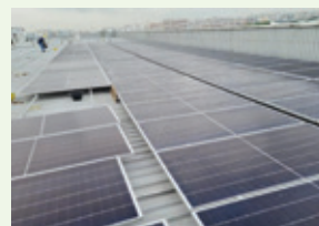
Solar panels at 37A Tampines Street 92, Singapore
