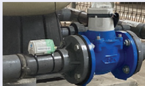
Smart water meter installed at Aperia, Singapore
